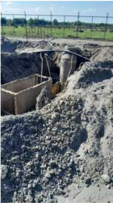
Worker without helmet in the trench
