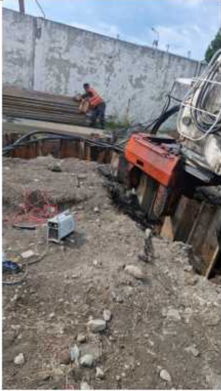
Worker without PPE in the trench
